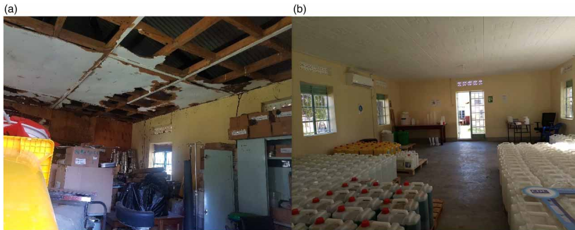
Figure 1 | Renovation and setup of the Kotido ABHR local production unit: (a) before renovation and (b) after renovation.
