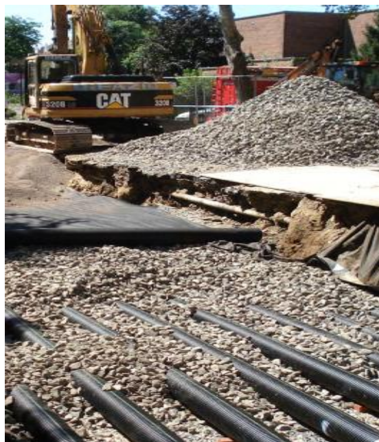
Figure 3-3 A perforated pipe system layout installation (New York City Department of Environmental Protection, 2012)
