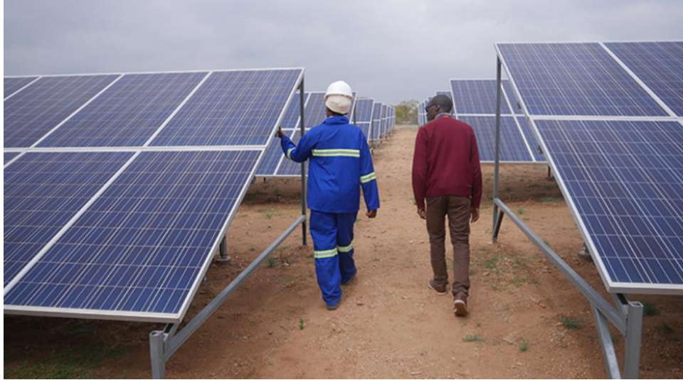
Figure 2: Solar panels that generate electricity for Mashaba mini-grid in Matabeleland South, Zimbabwe (Renewable energy catalyst for Zim’s socio-economic development n.d.)
