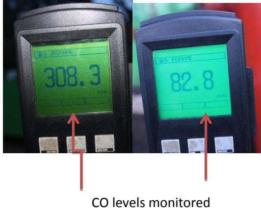
Figure 4: CO monitors reading at HPS start-up & at ambient running conditions
