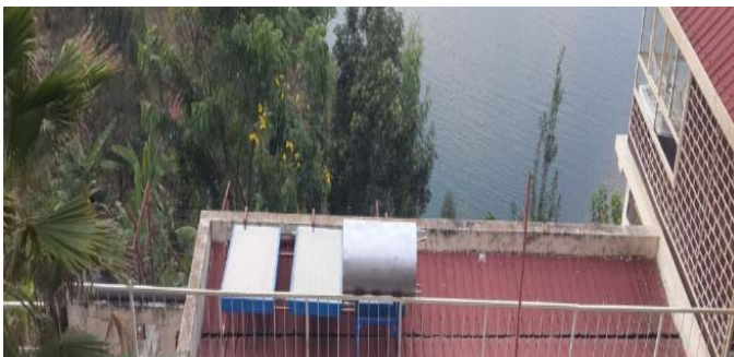
Fig.13.Already fixed solar water heater
