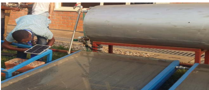
Fig.14.Smart meter system installation
