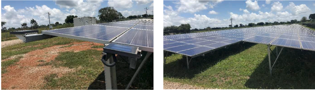
Fig. 3. Selected photos of Soroti solar power plant (Pictures: Ivan T Oloya).
