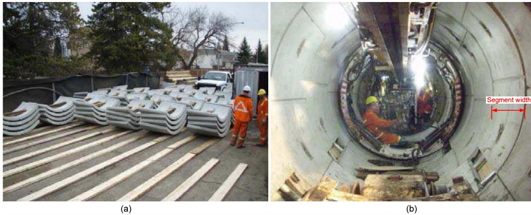
Figure 3: Segments for the project: (a) segments at the site; and (b) segments in the tunnel.
