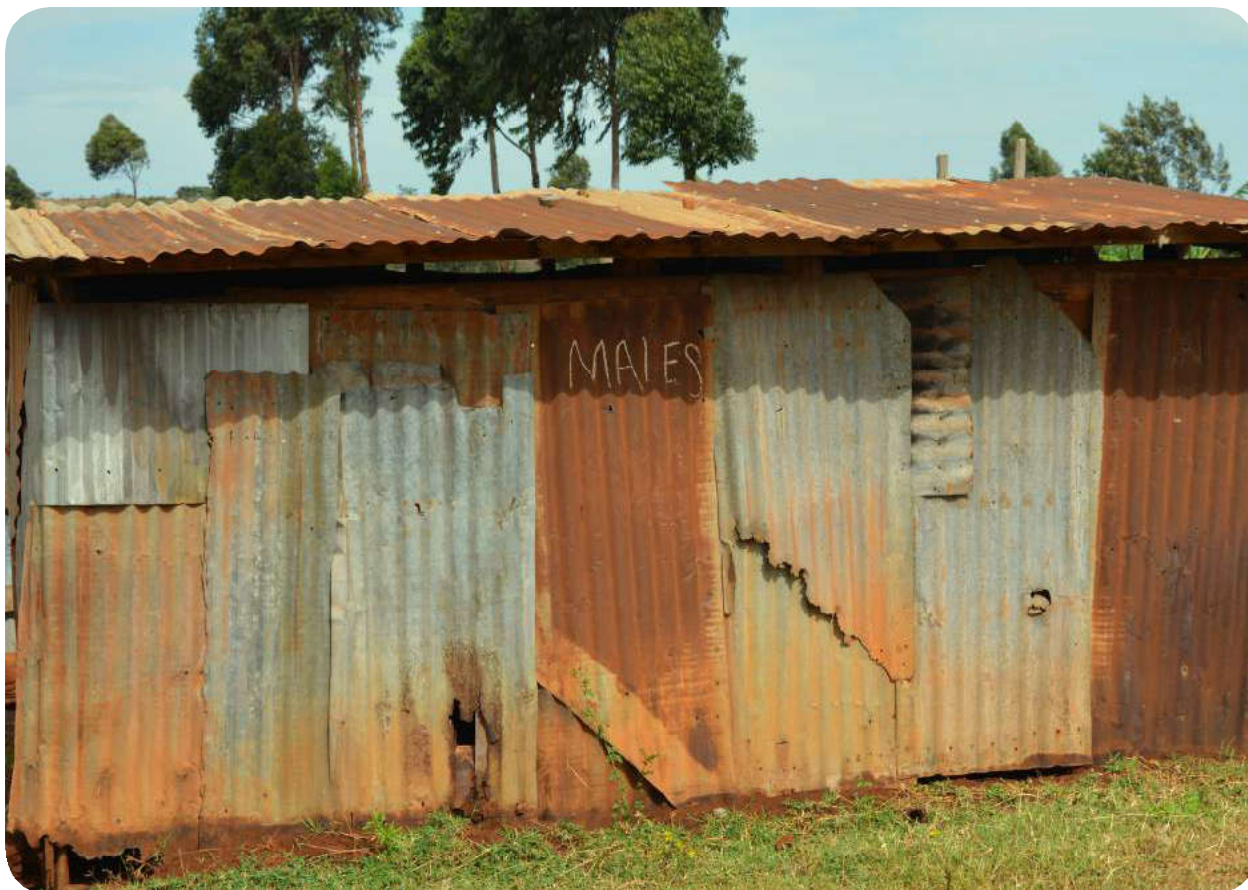
Very unsafe and unhygienic latrine at one of the private schools ISER visited in eastern Uganda
