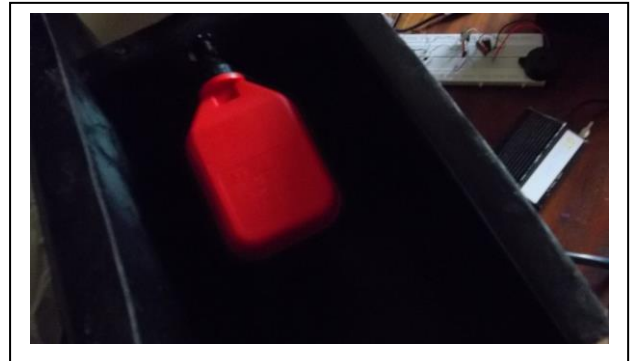
Fig. 3. Float switch inside a fabricated transformer compartment.
