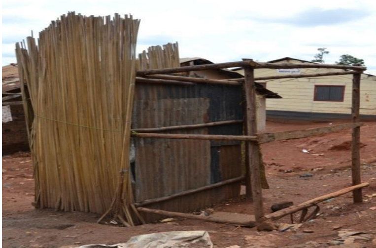
Figure 2.1: Sub-standard pit latrine in Kampala City
